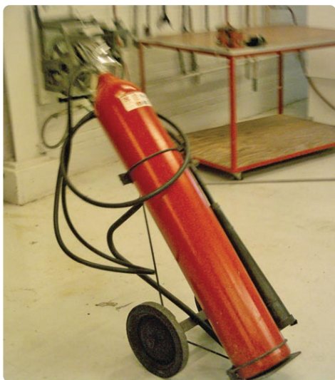
Figure 1-5. Carbon dioxide fire extinguisher.
