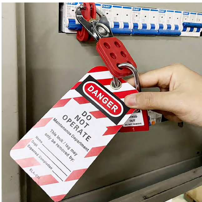
Figure 4-16. A circuit breaker panel with the system undergoing maintenance clearly tagged and locked out.
